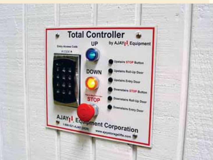
A lift controller panel.
