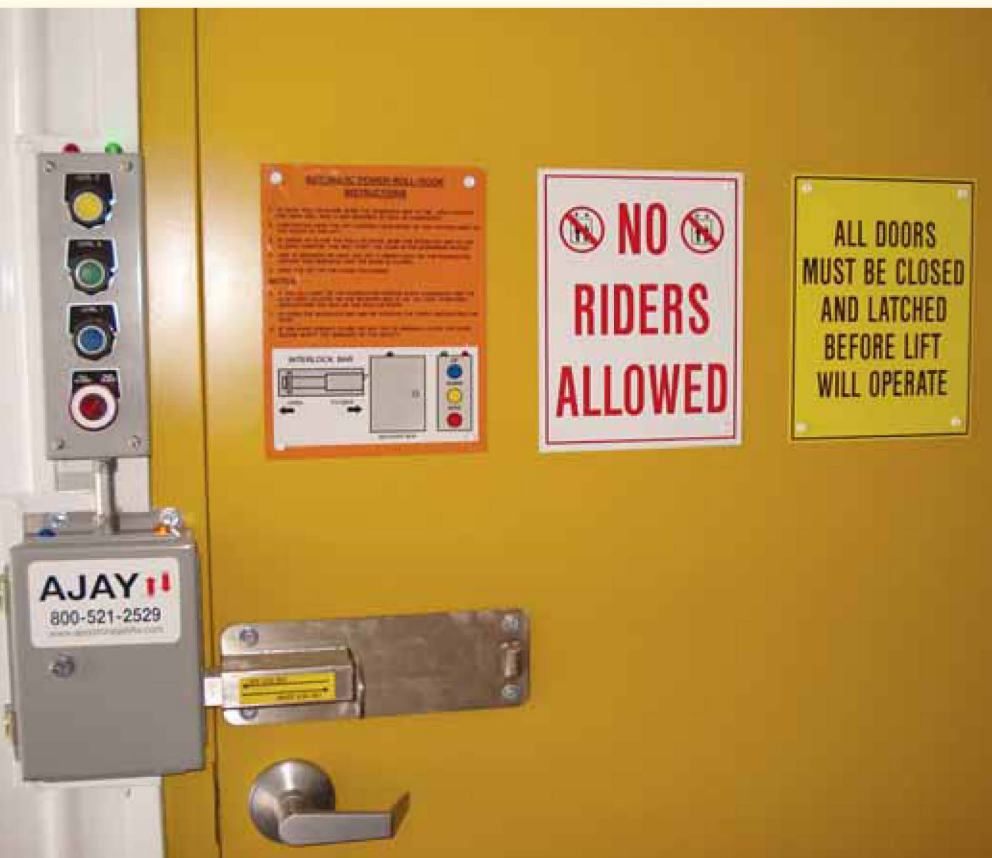
Signage is essential to tenant safety and proper lift use.
